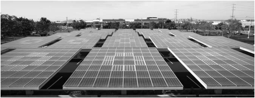
Figure 3-4: Kyocera “Solar Grove” – 25 Panels, 235 kW Total, 186 Vehicle Parking Lot.
