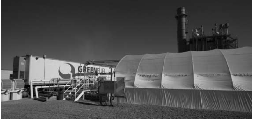
Figure 3-9: Pilot Engineering-Scale Microalgae Plant at the Redhawk Gas-Fired Power Plant in Arizona
